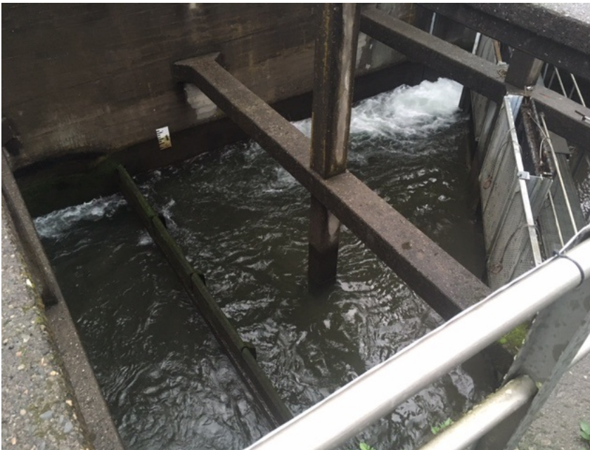
Figure 4. Actual water level at Cascades Island during the work period (15-17 Nov.) with UMT bulkhead in place.
